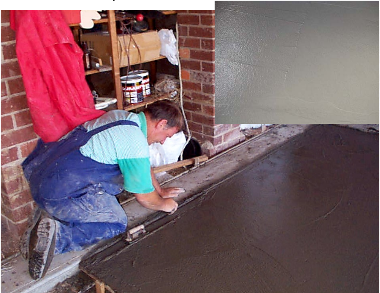
Figure 2 - Mike Burdon Finishing Off the Edges of a Low Slump Placed concrete with an Edging Tool. Insert – The Silky Finish Obtained
